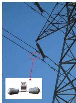
Vibration absorber in the transmission lines
